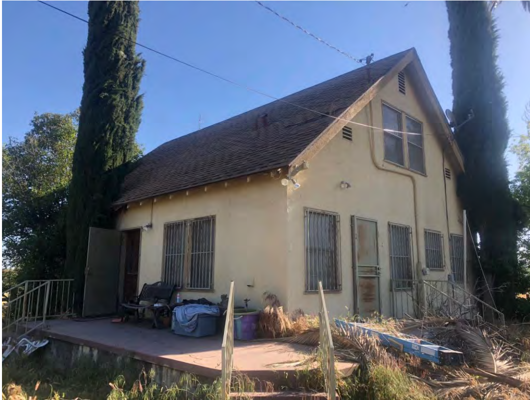
A) View looking northeast of the west and south facing facades. April 30, 2019. Acc. #201904fr2885
