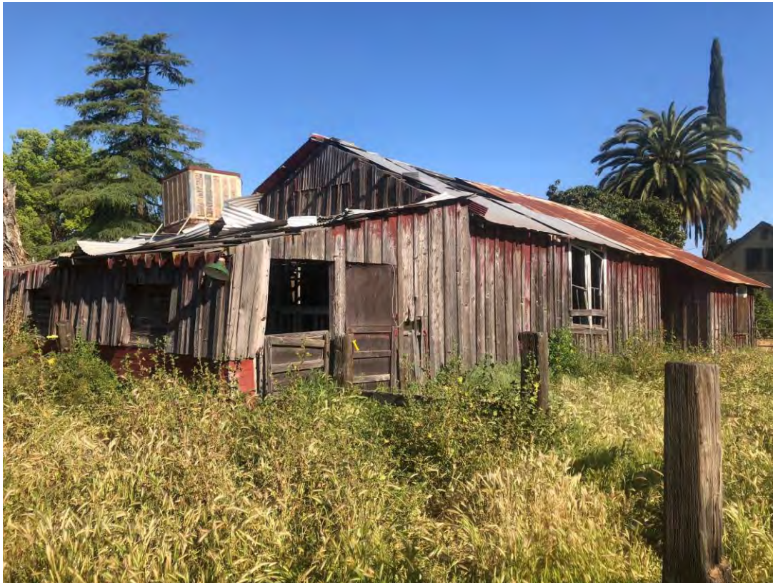
E) View looking northwest of the south and east facing facades of the barn. April 30, 2019. Acc. #201904fr2993
