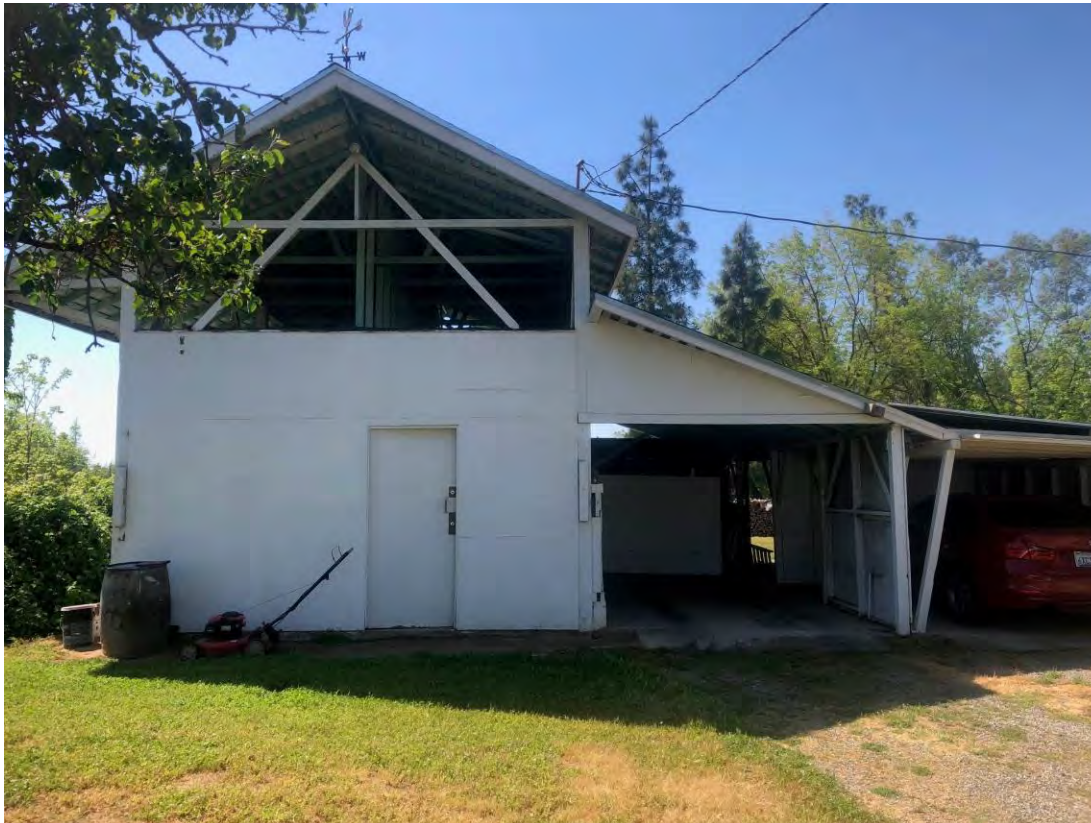
H) View looking south of the north facing side of Outbuilding #2. April 30, 2019. Acc. #201904fr3008
