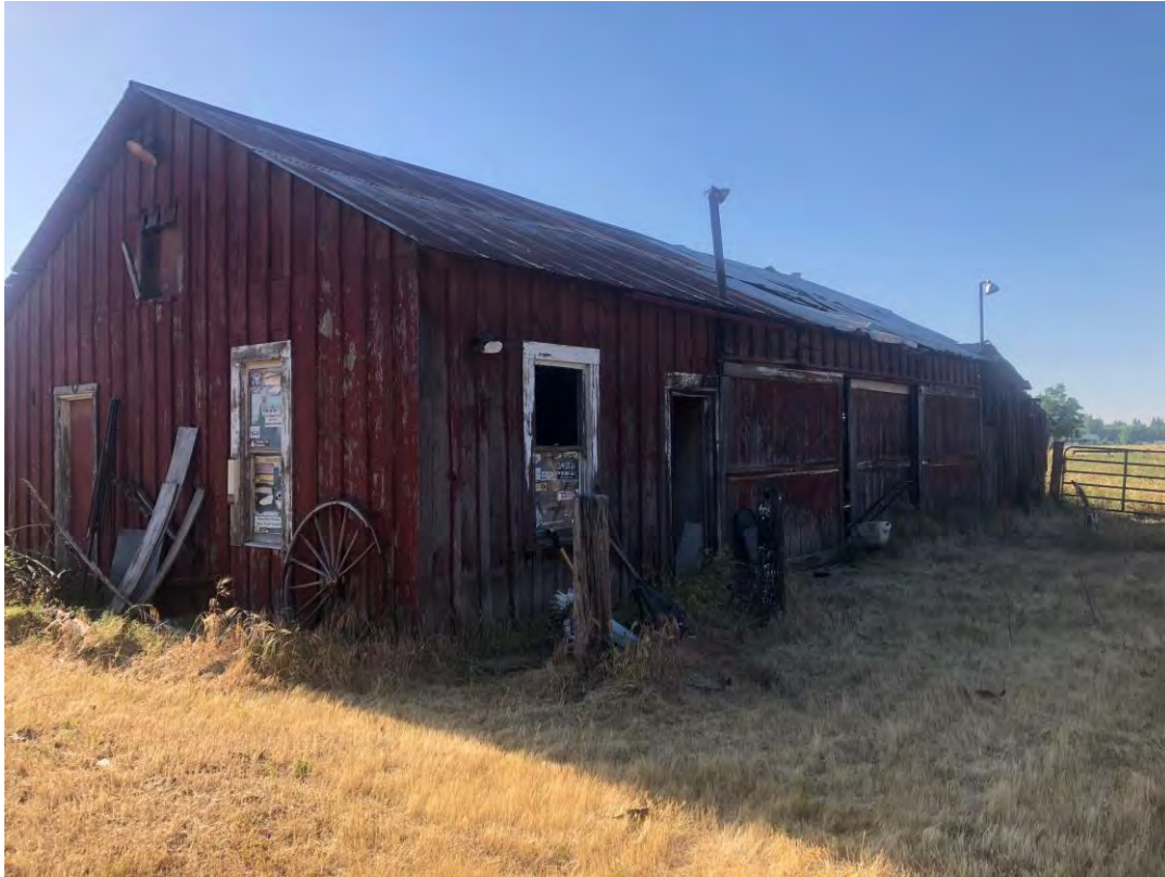
F) View looking southeast of the north and west facing facades of the barn. April 30, 2019. Acc. #201904fr2985
