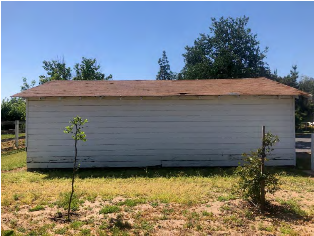
E) View looking south of the north facing side of Outbuilding #1. April 30, 2019. Acc. #201904fr3011
